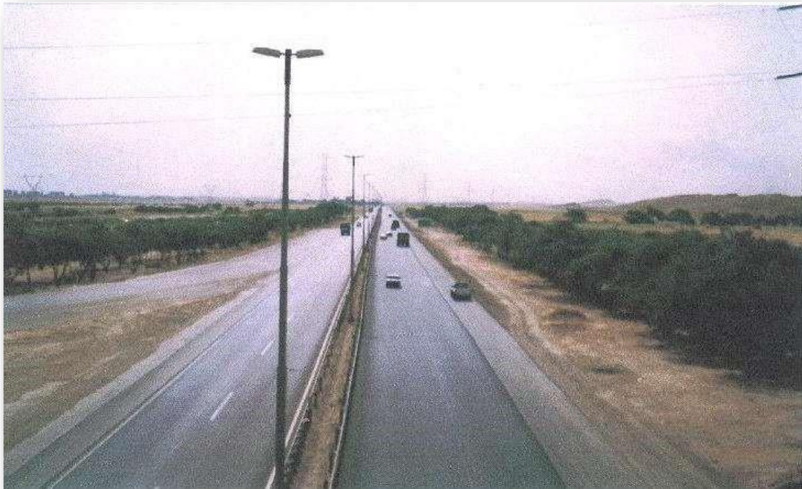
Figure-3 Repair and improvement of station 0 to 13 km of Ahwaz-Mahshahr path, Khuzestan road and transportation (1385)
