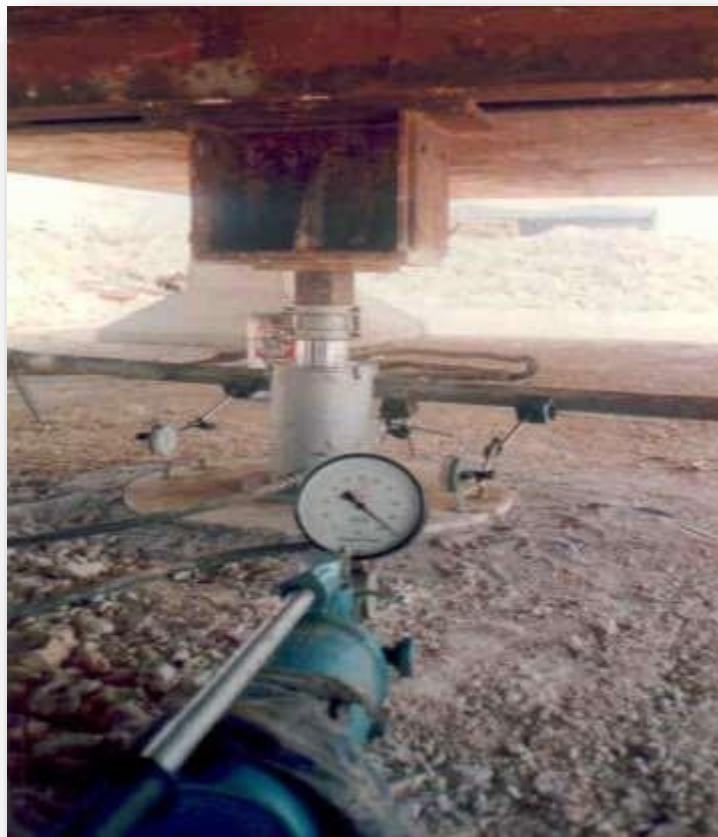
Figure-5 View of the plate loading test on the Caspian Sea site, Sadra Company (1381)
