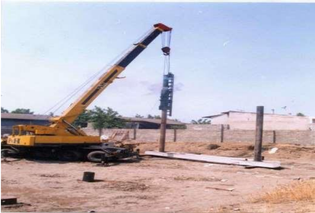
Figure-1 Design of foundation system, compaction and piling operations of 12-storey residential complex in Babolsar (1382)
