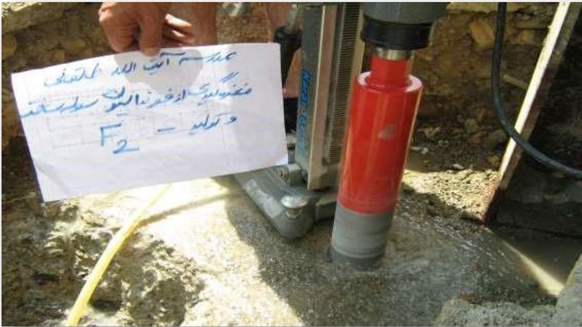
Figure-21 Concrete core test of Ayatollah Taleghani concrete Foundation, District 5, Tehran, Equipping Tehran schools (1387)
