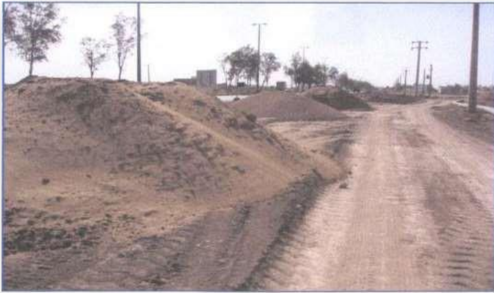
Figure-9 Prepare of materials for construction of two polyethylene pipelines along the passage of site B, Arvand Free Zone, Ahvaz (1388)
