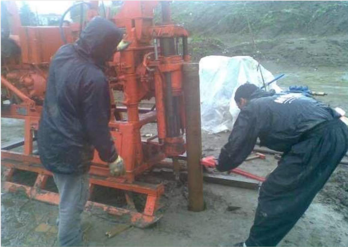
Figure-7 Drilling operations in the 34-storey residential tower project of Sika, Chalous (1389)
