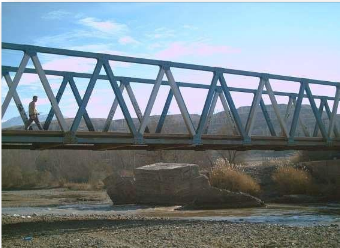
Figure-4 Studies and design of reinforcement of Amiran Bridge, General Department of Roads and Transportation of Tehran Province (1385)
