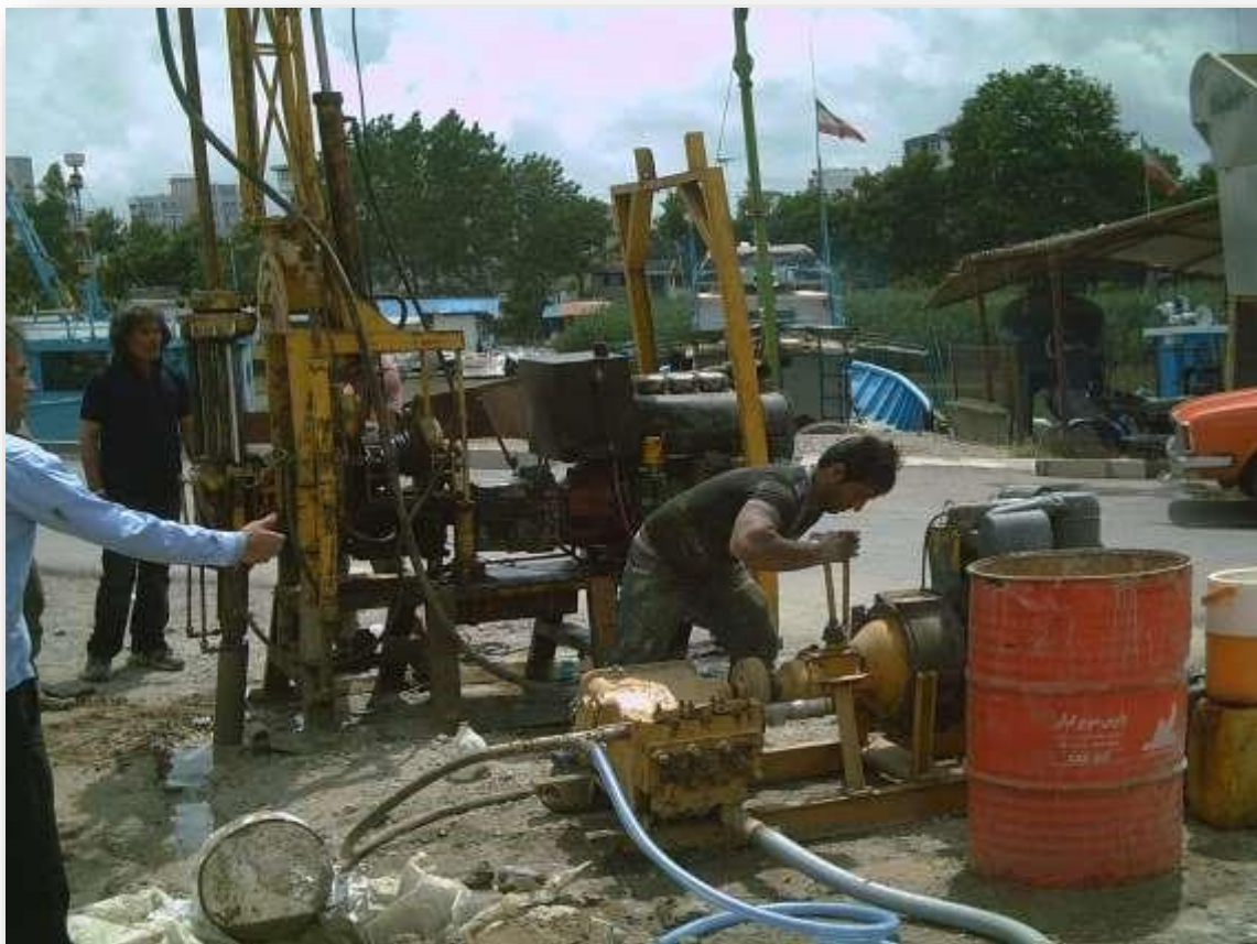
Figures-11 & 12 Excavation of machine trial boreholes in the fourth bridge of Babolsar (1390)
