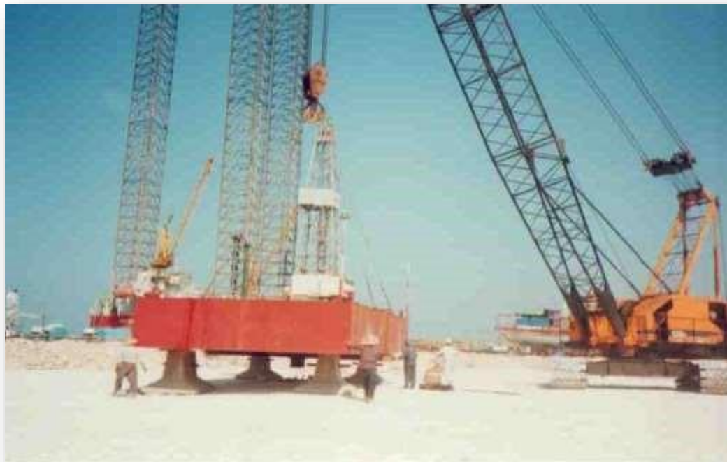
Figure-6 View of the cranes installation to perform plate loading test, Sadra Company, Caspian Sea Complex (1381)
