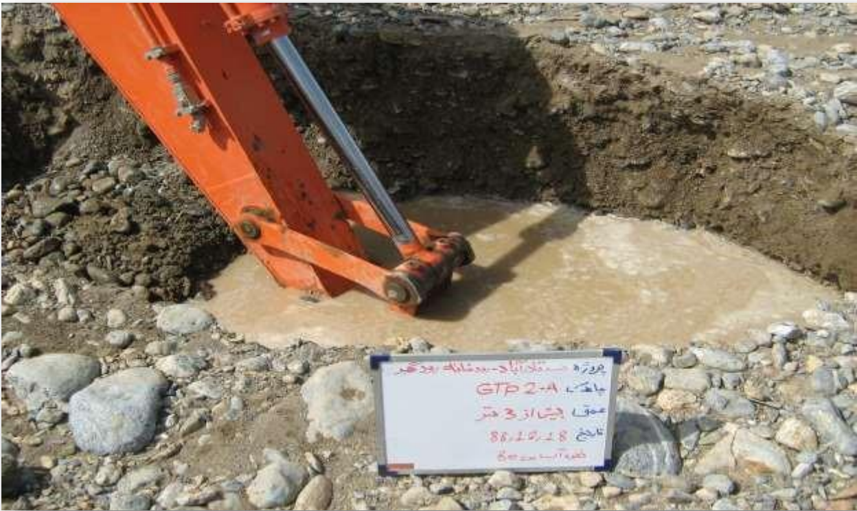
Figure-3 Geotechnical investigation of Qaderabad Dam, Sistan and Baluchestan Regional Water joint-stock Company (1388)
