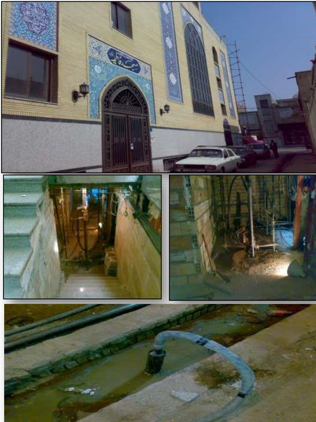
Figure-27 Performing micro piles in the project of improving the foundation of Fatemeh Mosque located in Qala-e-Marghi, District 17 Municipality (1387)
