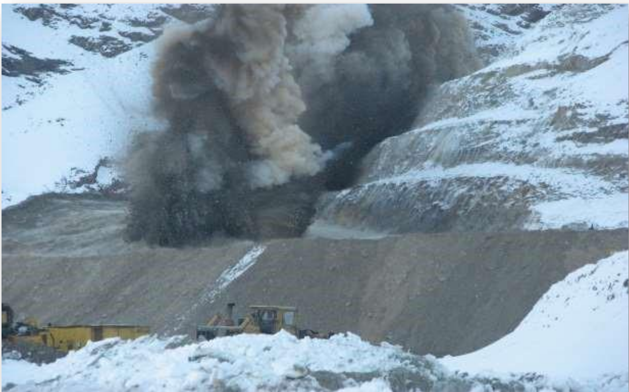
Figure-8 Explosive operation at station 4+800 km of Yalrud-Sorkhak axis, Ministry of Roads and Transportation (1388)
