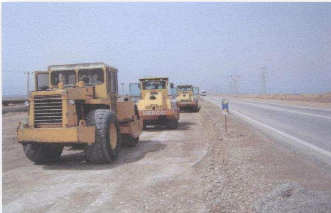
Figure-4 Execution operation of the subbase layer of Abadan-Mahshahr axis 10 km length, National Company for Refining and Distribution of Petroleum Products (1386)
